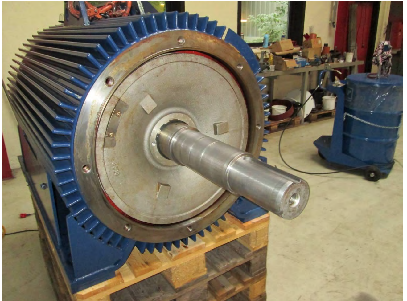
Bearing exchange generator DE
