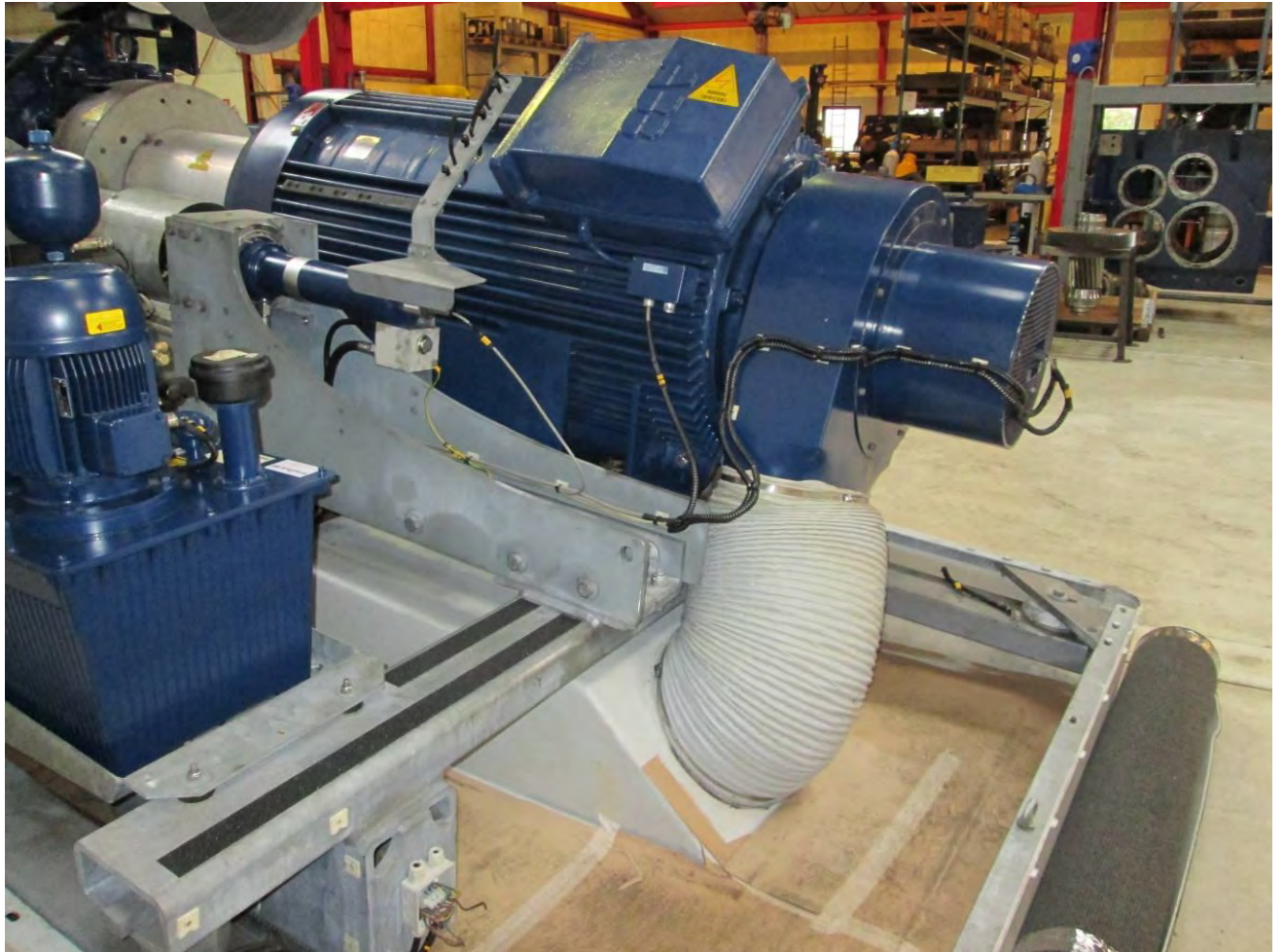
Generator mounted in turbine.
